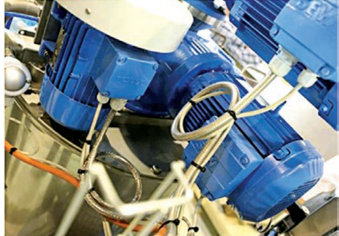
Loops along cables trap dirt and are tough to clean and should be avoided in food production
