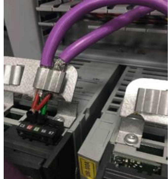
VFD shielding corrected
