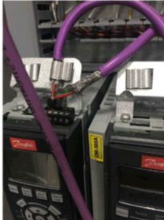
VFD shielding not as per standards
