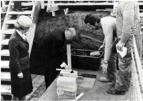
Ursula Ida and Oskar Lapp lay the foundations for today's Lapp cable factory building in Oskar-Lapp-Straße 5
